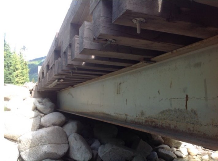
missing some deck clips
